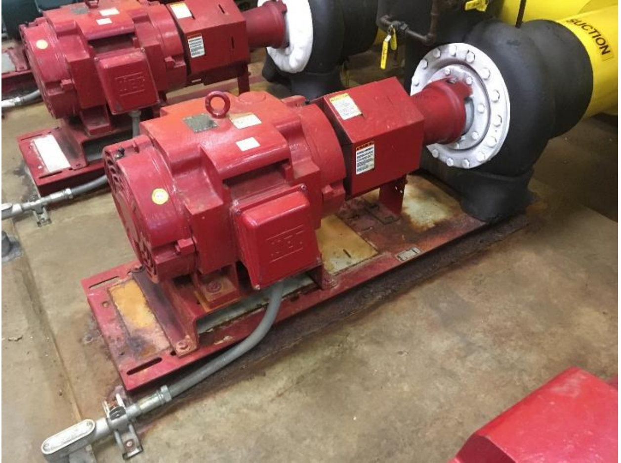
Brine pumps (note corroded steel base against concrete pump base)
