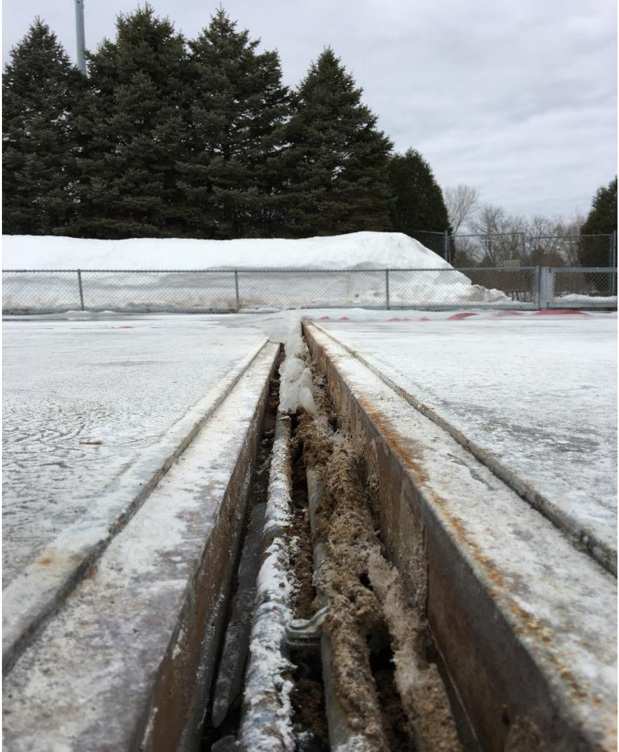
Expansion joint heaving from excess water getting beneath rink slab and freezing
