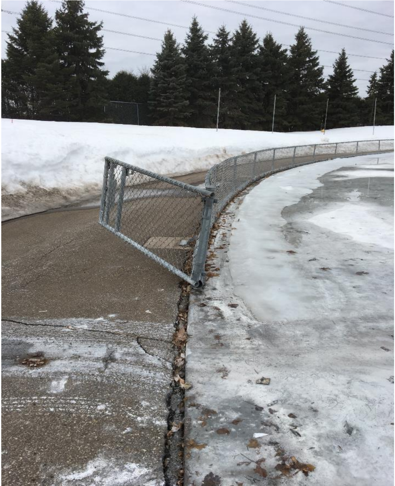
Perimeter pavement damage and skewed fence alignment from rink slab movement
