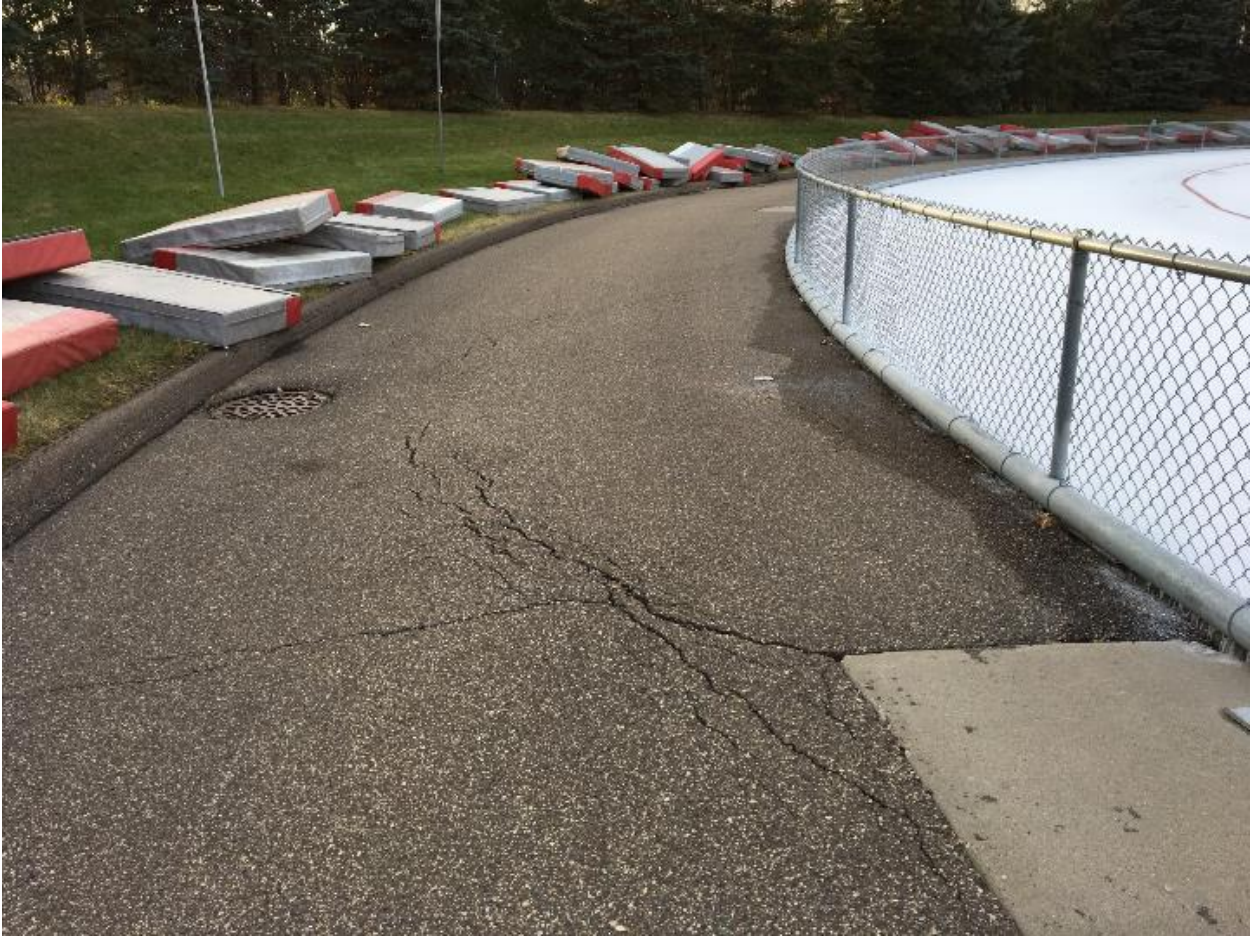
Perimeter pavement damage adjacent refrigeration slab due to refrigeration slab movement
