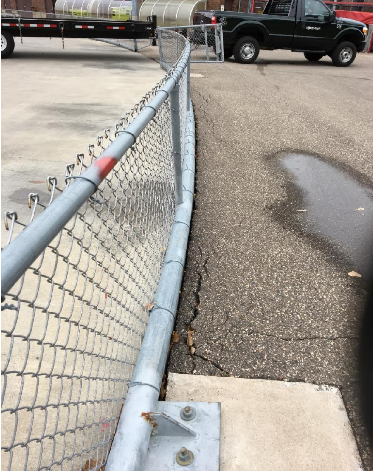
Skewed perimeter fence and pavement damage at southeast corner of rink slab
