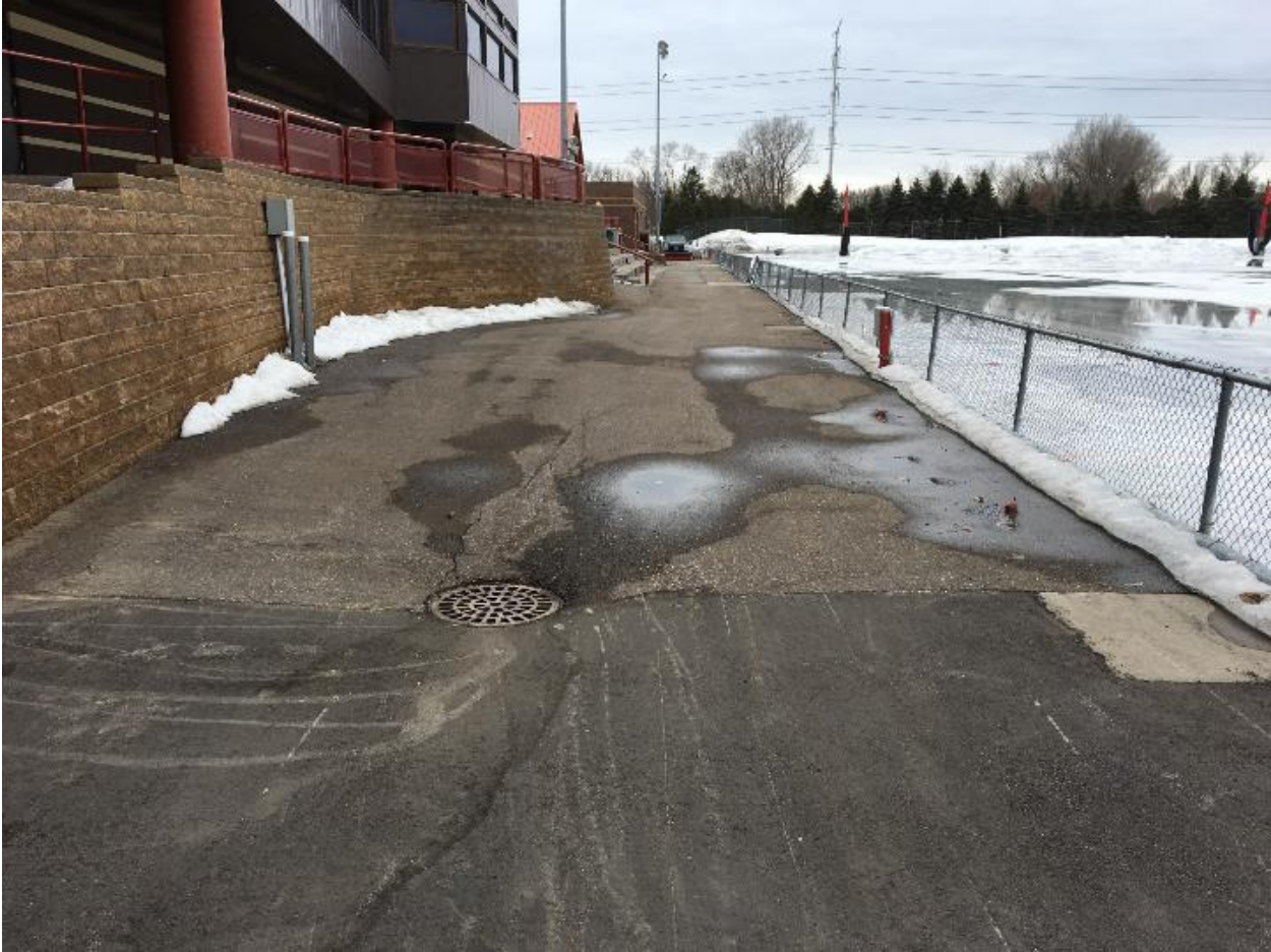
Poor perimeter pavement drainage
