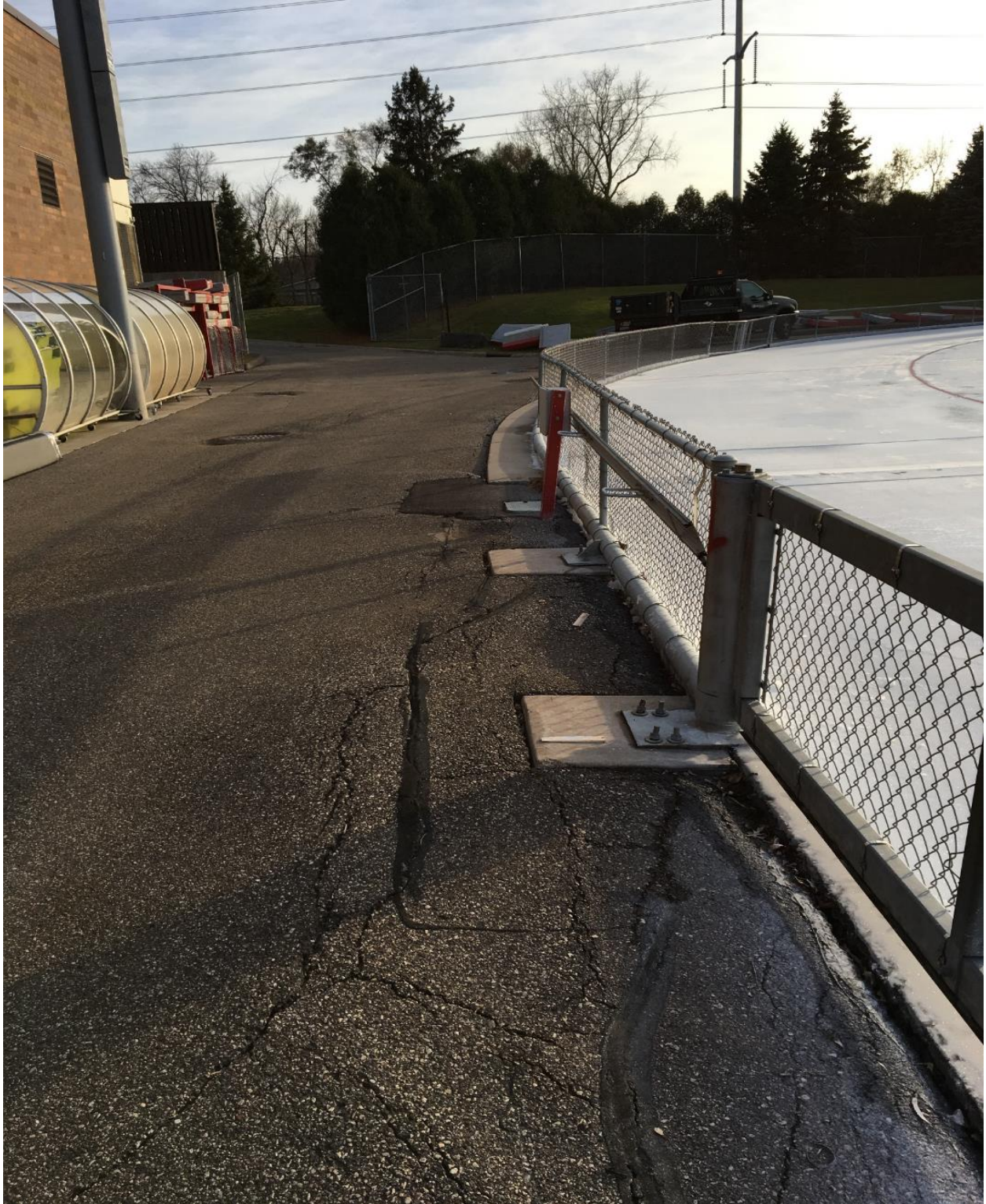
Perimeter pavement damage adjacent refrigeration slab due to refrigeration slab movement
