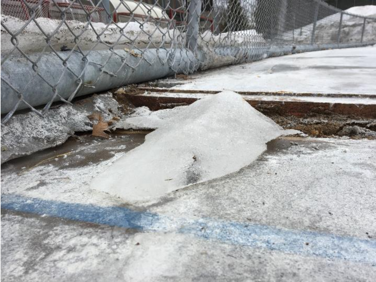
Frost heave in southeast expansion joint due to water infiltration and freezing below ice slab
