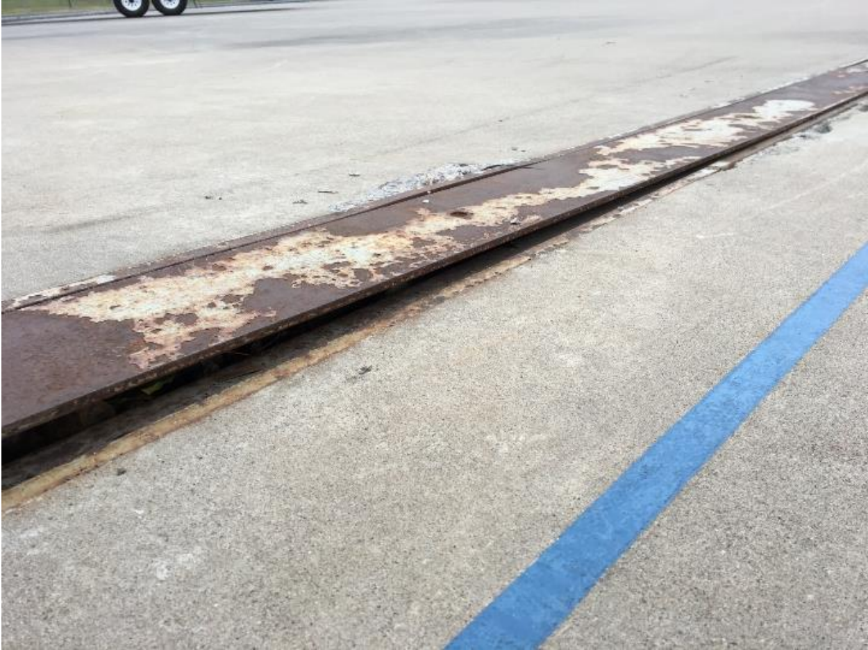
Lifting expansion joint plate at southeast corner of rink near end loop header
