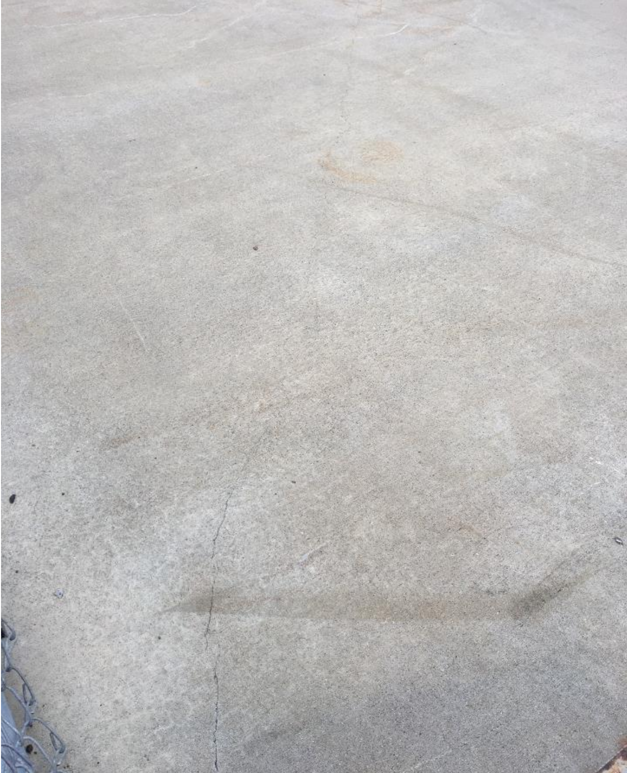
Hairline cracking of ice rink slab near southeast corner of rink on end loop
