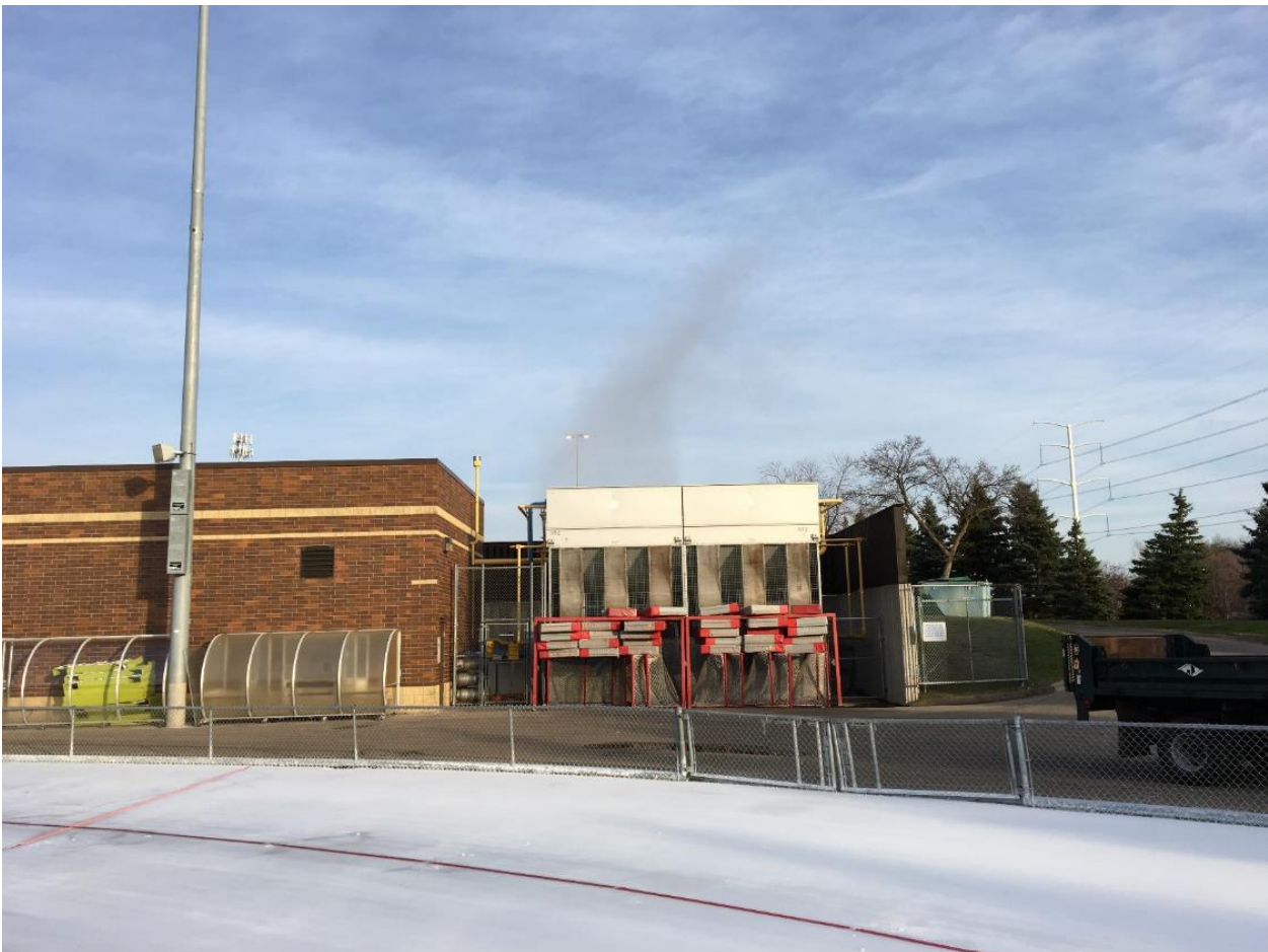
Evaporative condenser adjacent refrigeration room
