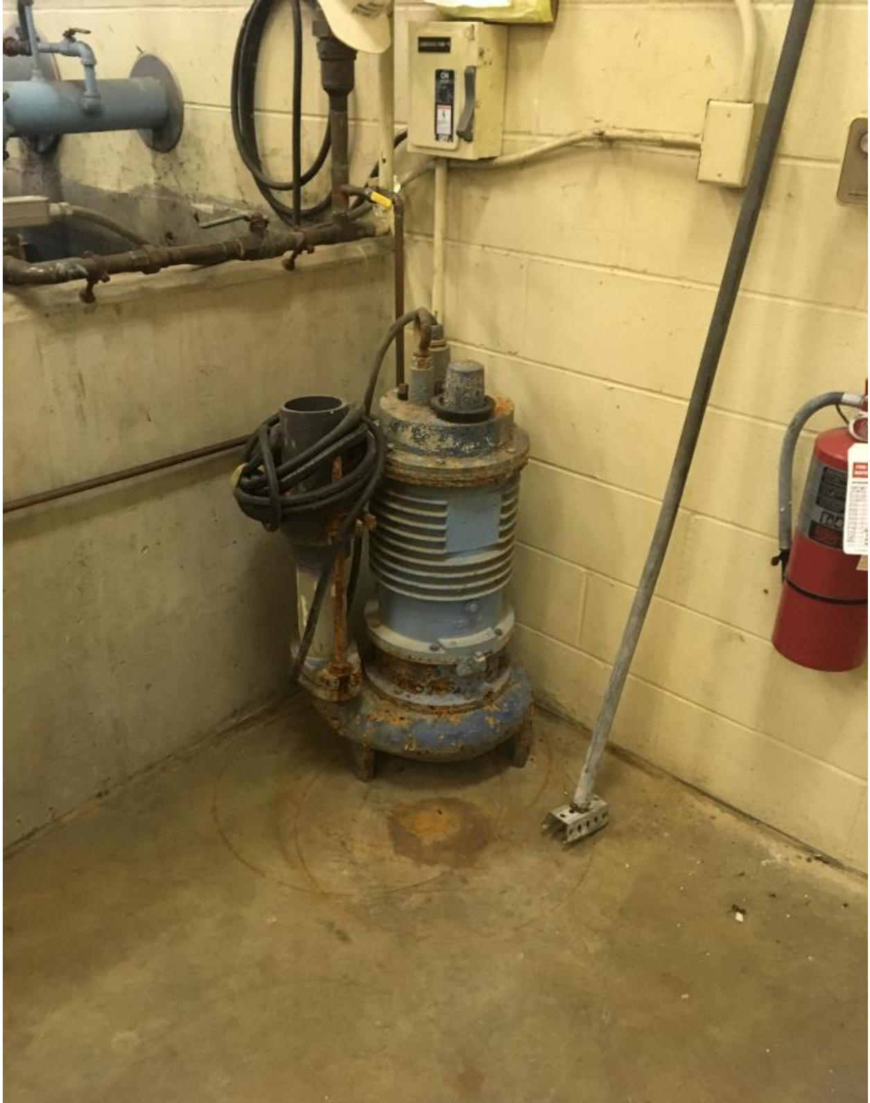
Failed condenser pump from remote evaporative condenser sump
