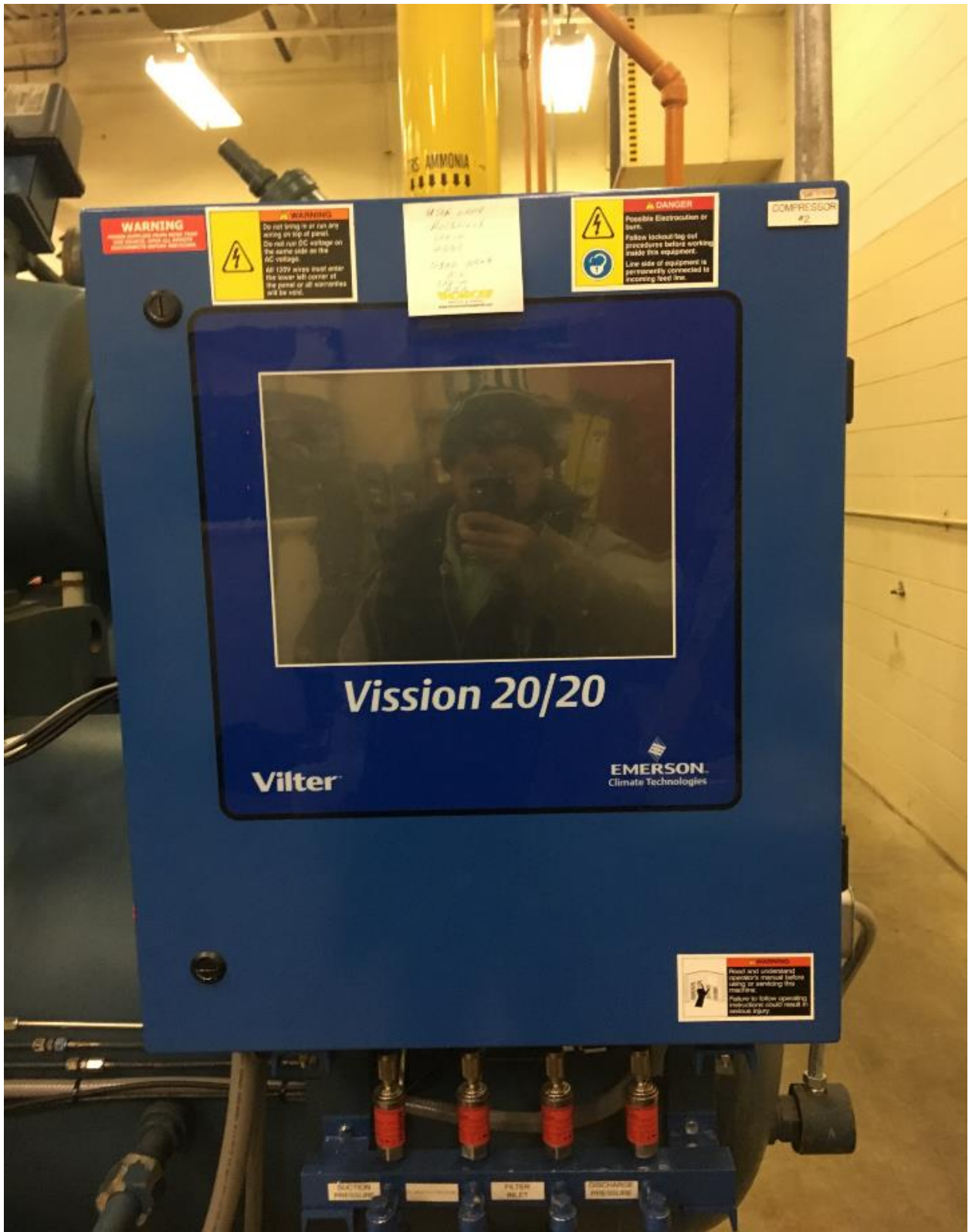
Newer replaced Vision 20/20 Vilter microprocessor control for compressors
