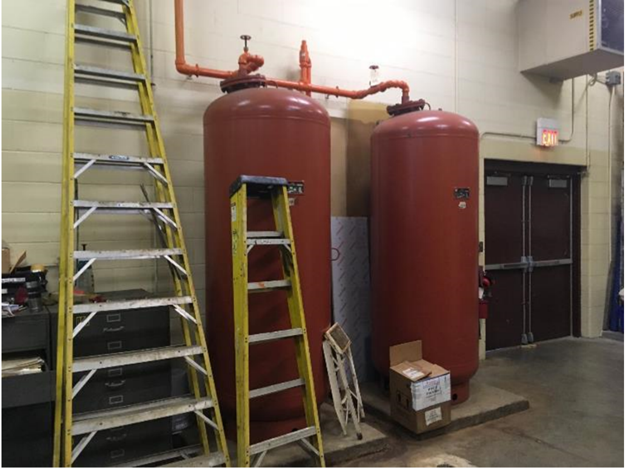
Bladder expansion tanks (bladder on one tank has failed)
