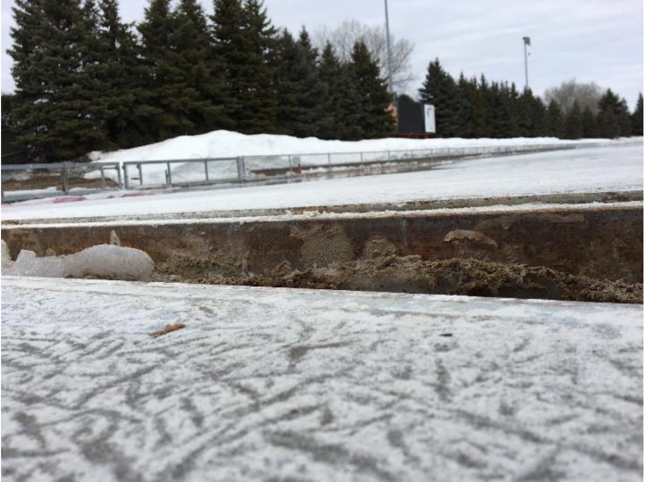
Expansion joint heaving from excess water getting beneath rink slab and freezing
