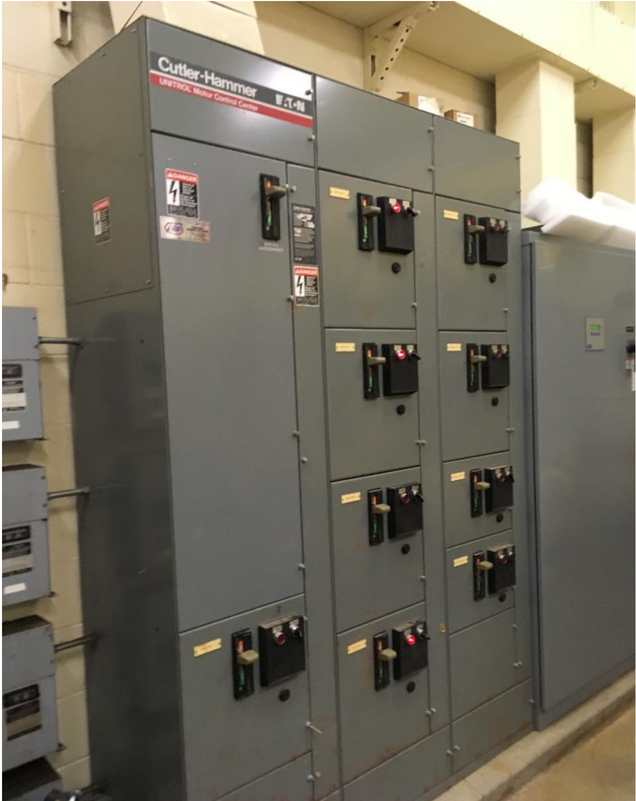
Motor control center for refrigeration system equipment
