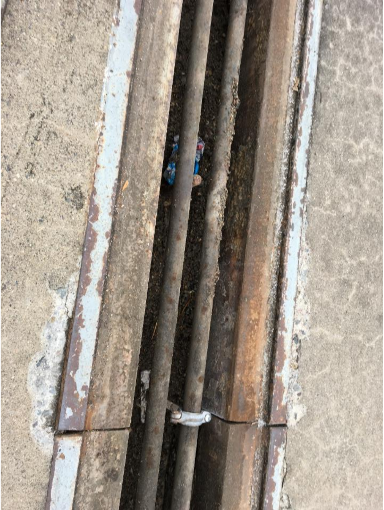
Deteriorating expansion joint channel at northwest corner of slab near end loop
