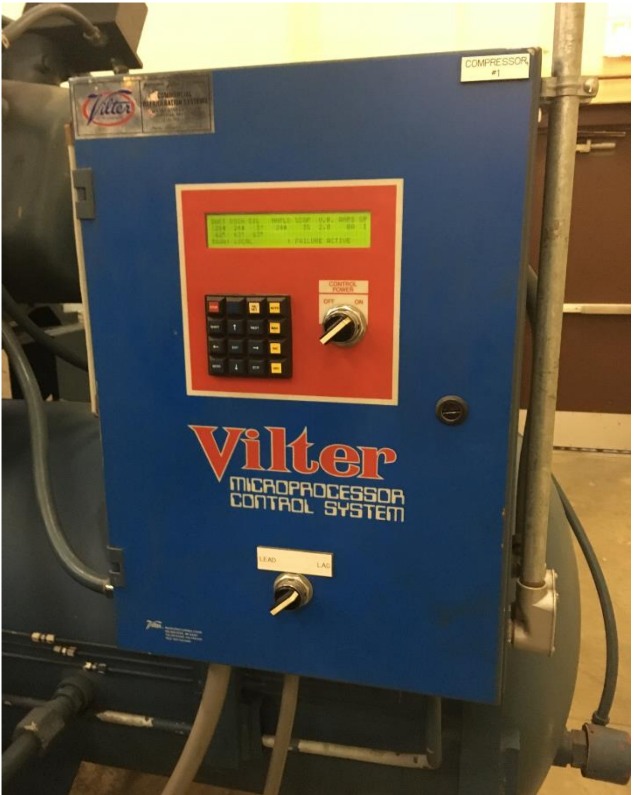
Outdated original Vilter microprocessor control for compressors
