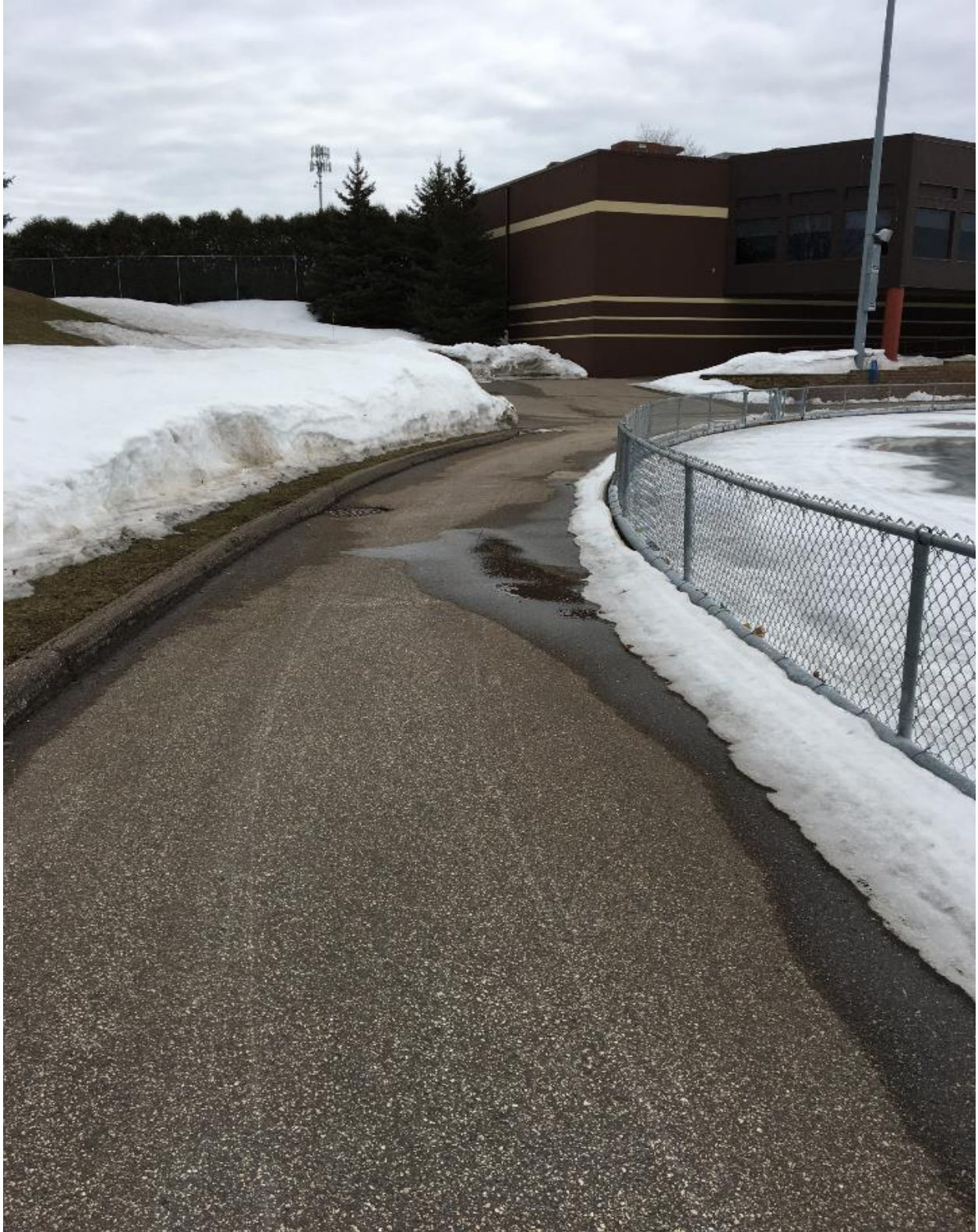
Poor perimeter pavement drainage
