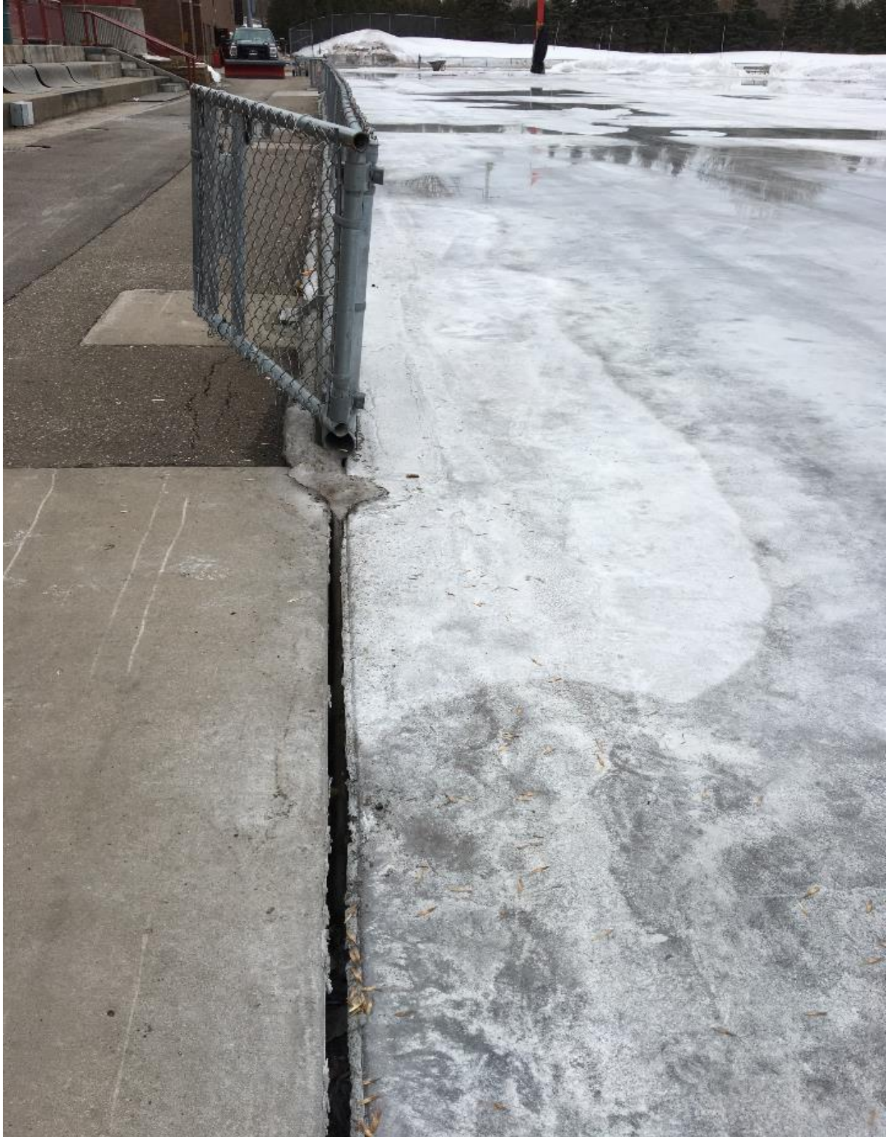
Poor perimeter drainage from ice slab movement
