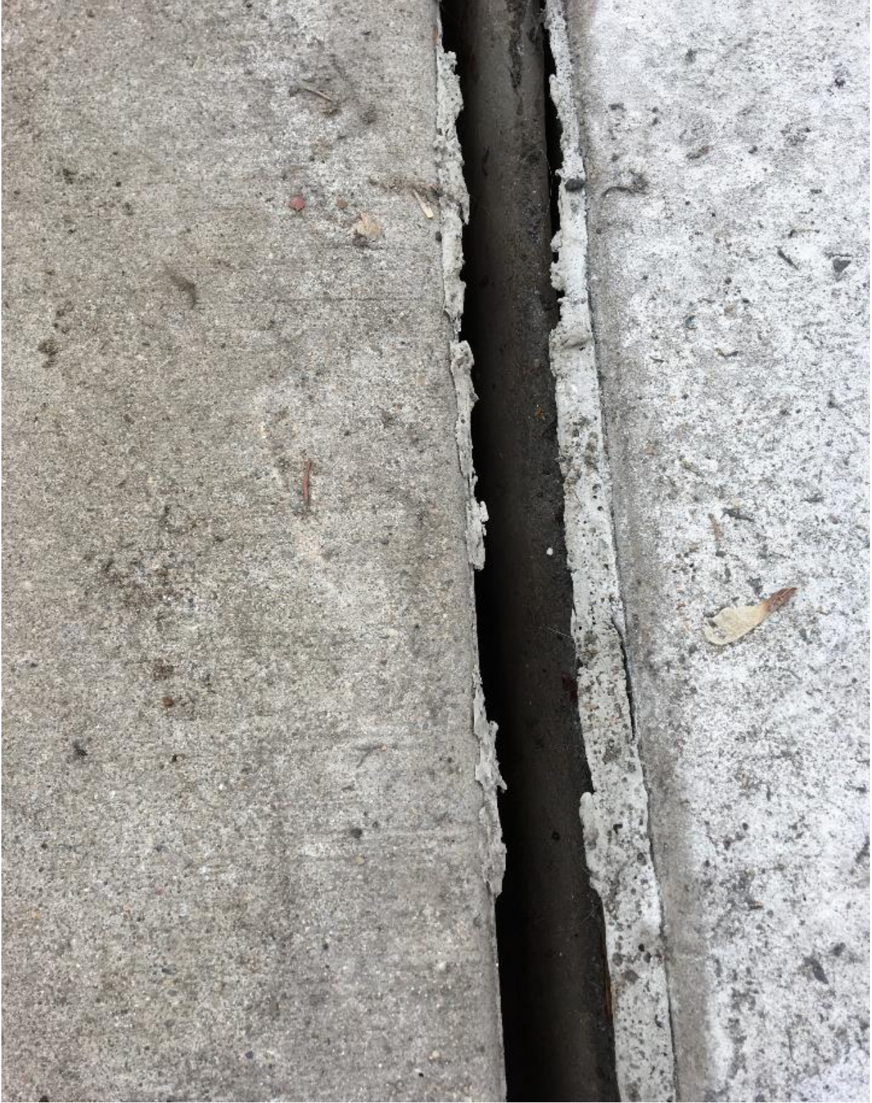
Poor perimeter drainage from ice slab movement
