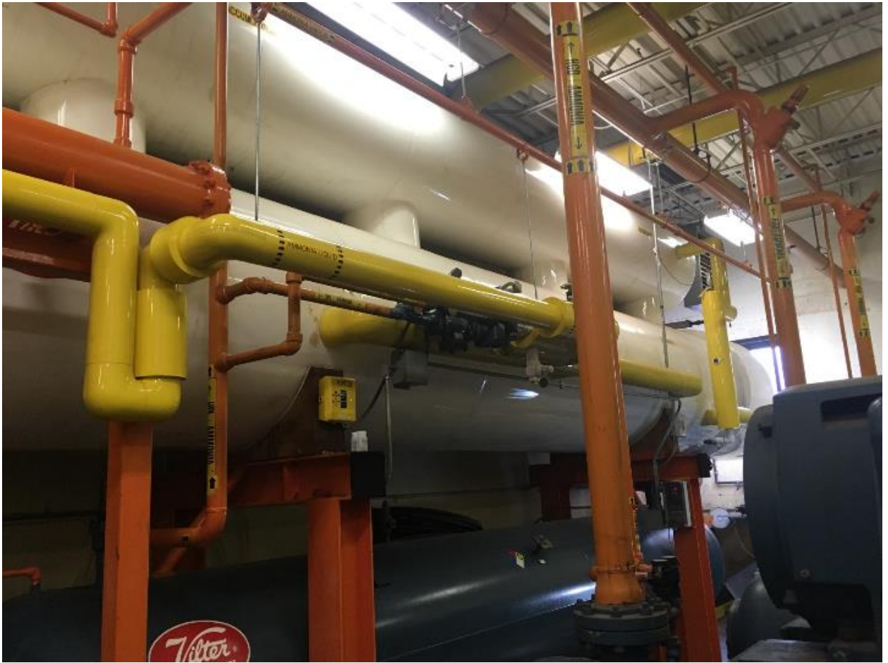
Chiller (above) and high-pressure receiver (below)
