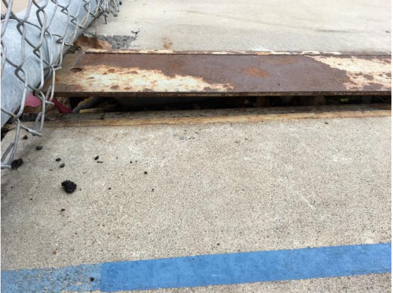
Lifting expansion joint plate at southeast corner of rink near end loop header
