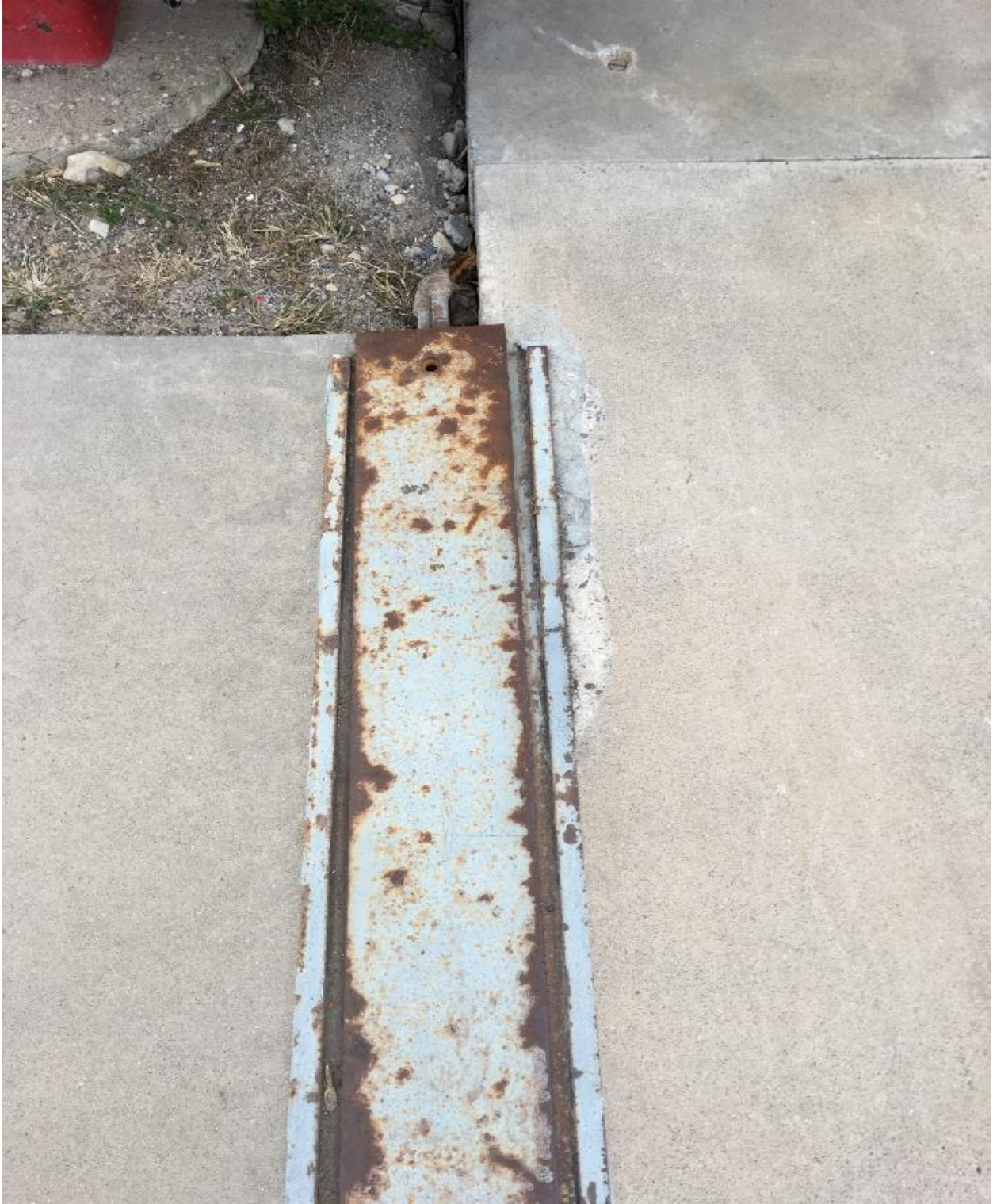
Concrete damage adjacent expansion joint due to wrong expansion plate use
