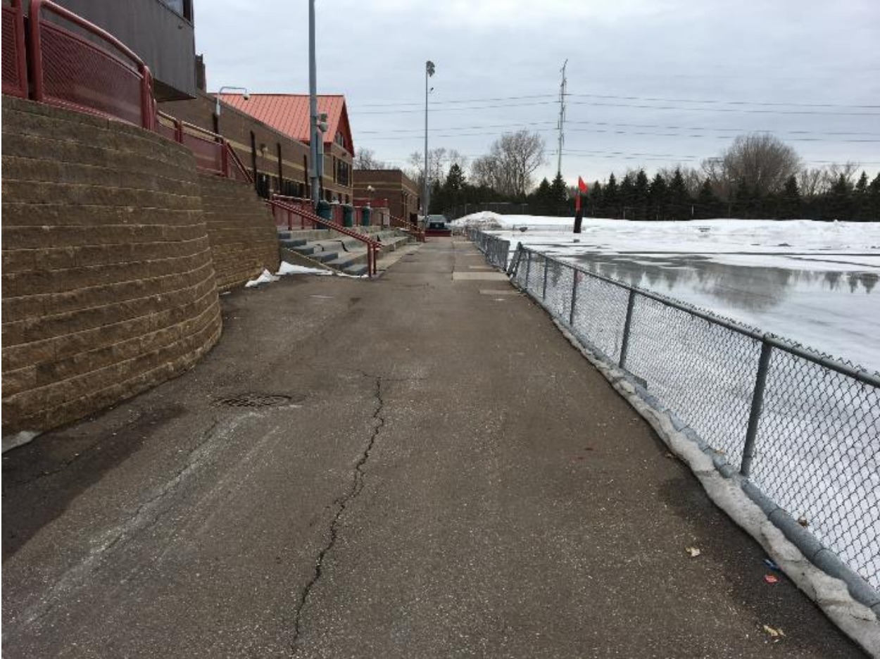
Poor perimeter pavement drainage
