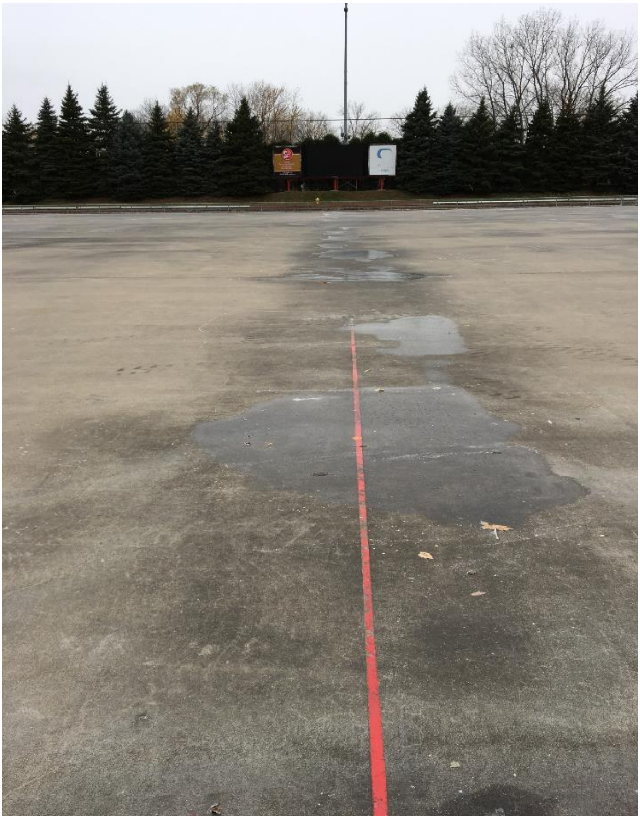
Settled center header for bandy rink
