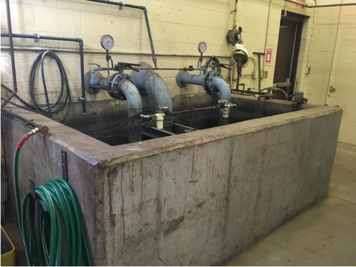
Remote condenser sump in refrigeration room
