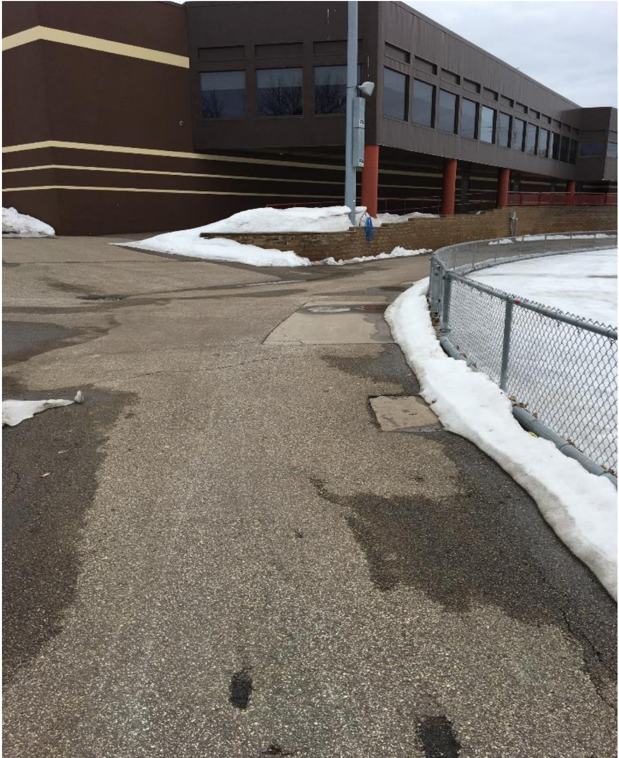
Poor perimeter pavement drainage
