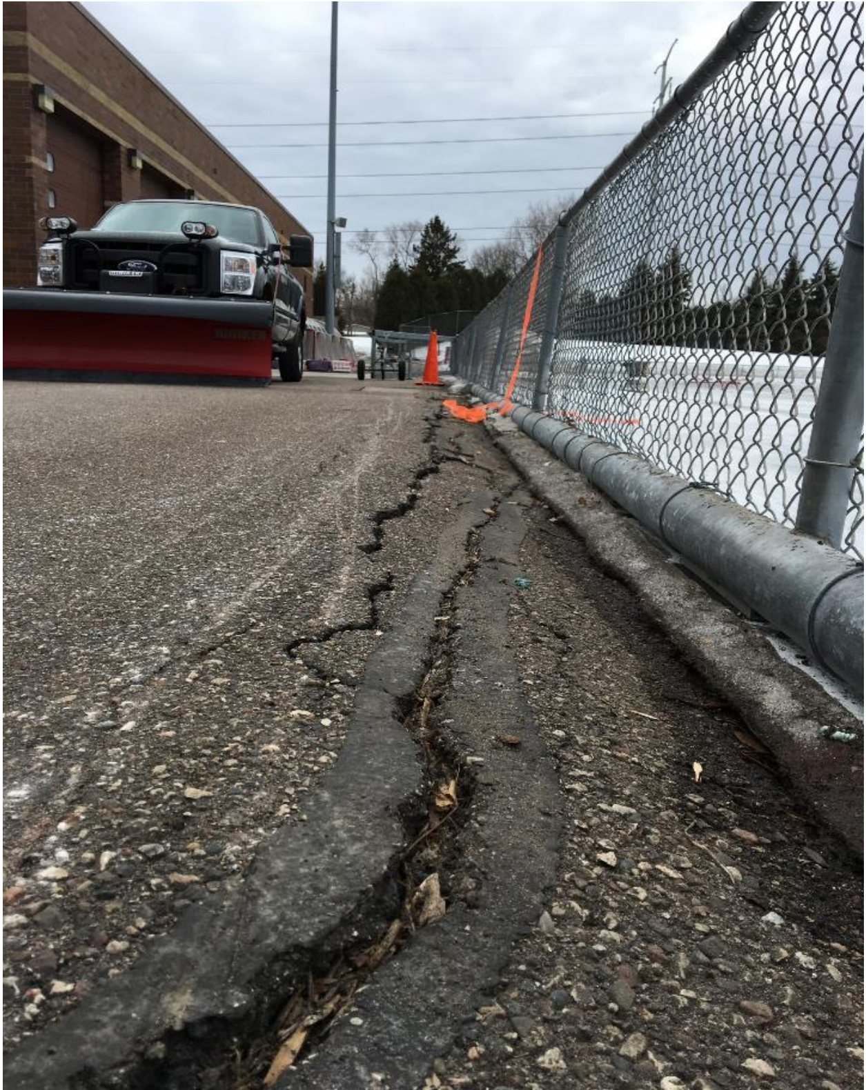
Perimeter slab damage and poor perimeter drainage due to ice slab movement
