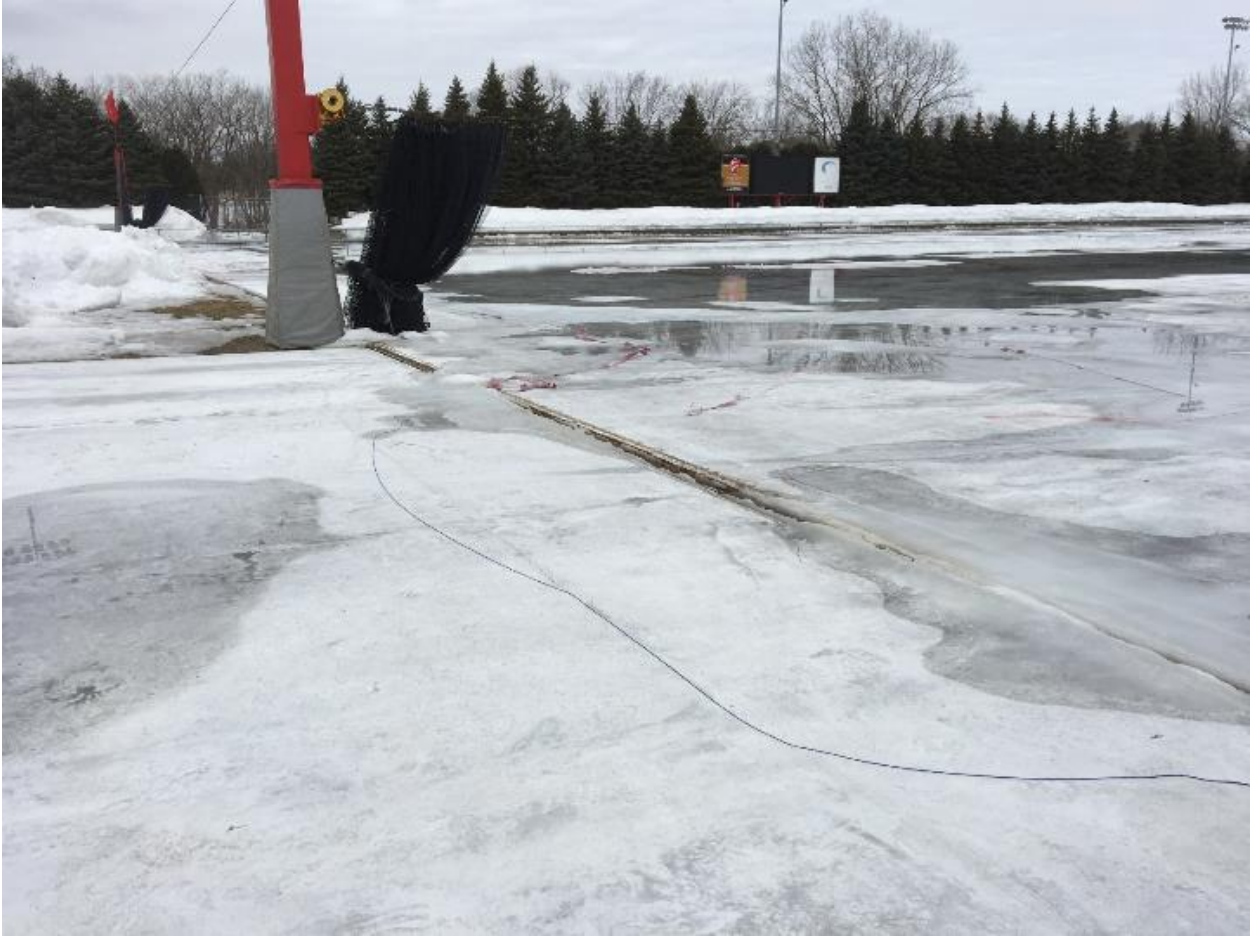
Expansion joint heaving from excess water beneath rink slab
